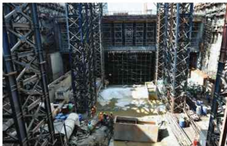
A Metro station being constructed at Mumbai’s BKC. The area has seen a sharp rise in dust pollution due to construction of infrastructure and residential buildings
